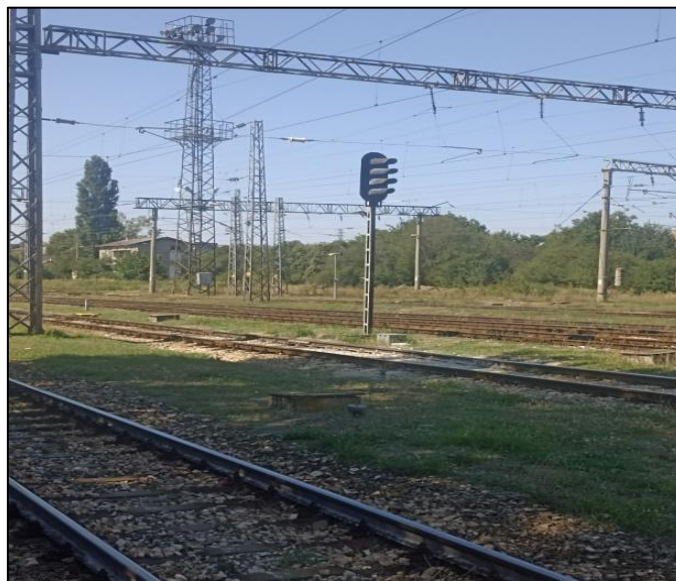
Fig. 4. Catenary and Traffic Light
