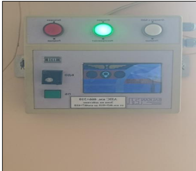
Fig. 5. Automatic Crossing Device (APU) Panel
